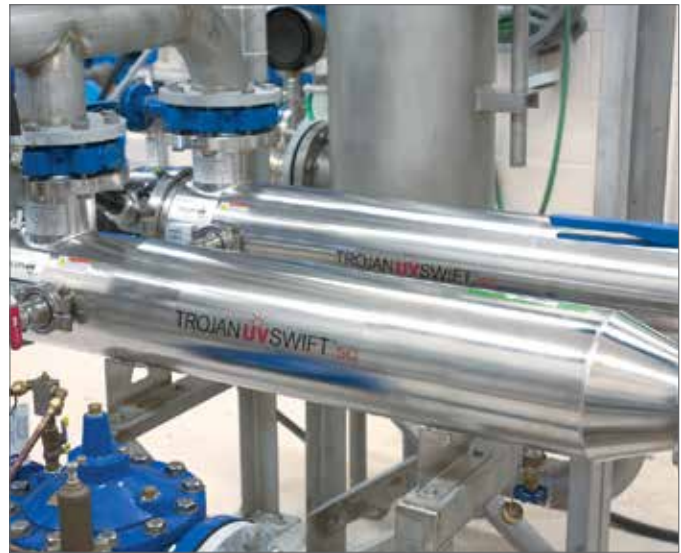
Drinking water disinfection in Neustadt, Ontario - 47 m 3 /hr (208 GPM)
