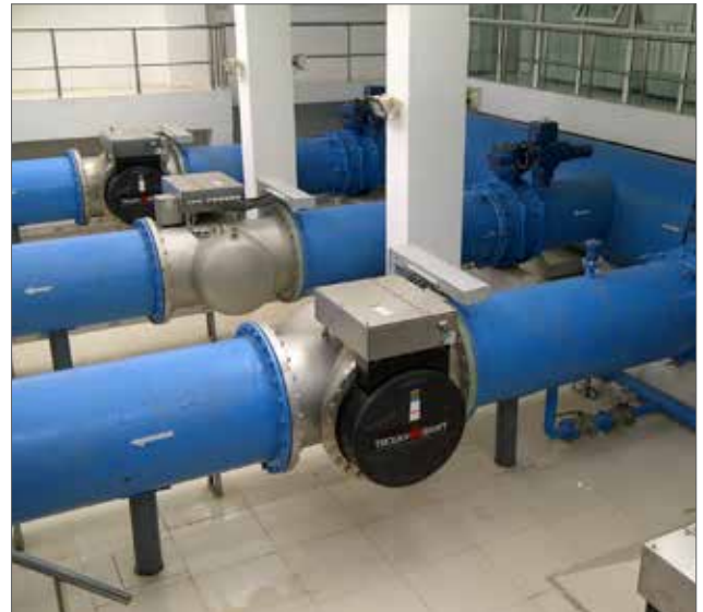
Drinking water disinfection in Tianjin, China – 6,250 m 3 /hr (40 MGD)
