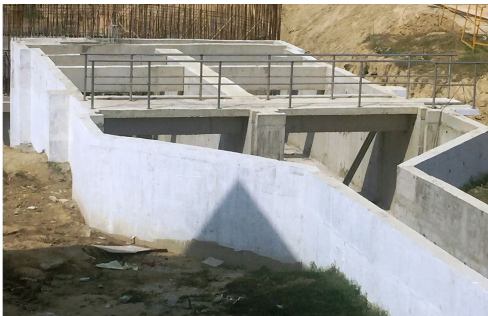
These concrete channels now house the TrojanUV3000Plus disinfection system at the Varanasi Sewage Treatment Plant.
